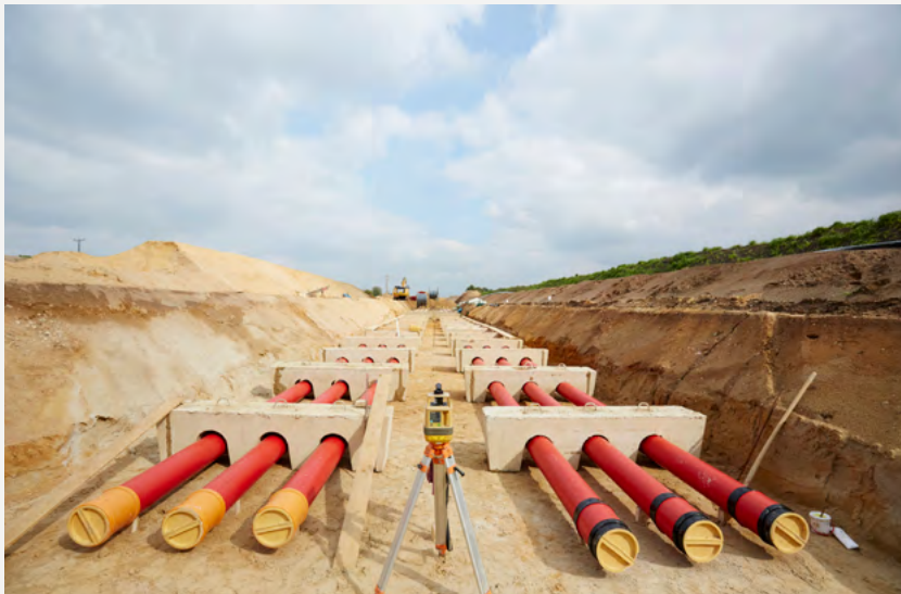
Rhein-Main-Link project. Image by Amprion
