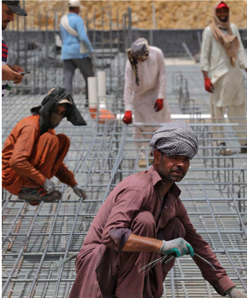
Labourers work on a steel mesh at a construction site in Saudi Arabia's capital Riyadh on May 23, 2022 during a heat wave. © FAYEZ NURELDINE/AFP via Getty Images
